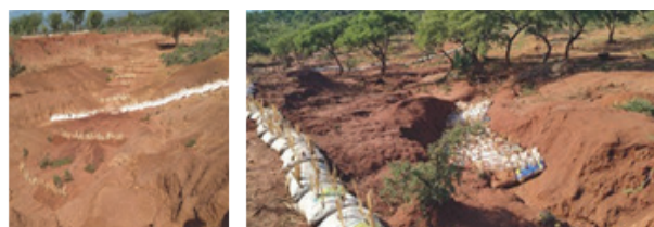
Gullies being rehabilitated at the Livestock Café sites in Chepareria Ward (Photo by M. Nyaga)
