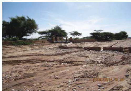
Plate 100: The sluice gates at Beer River should be continuously maintained. Photo Source FAO Manual
